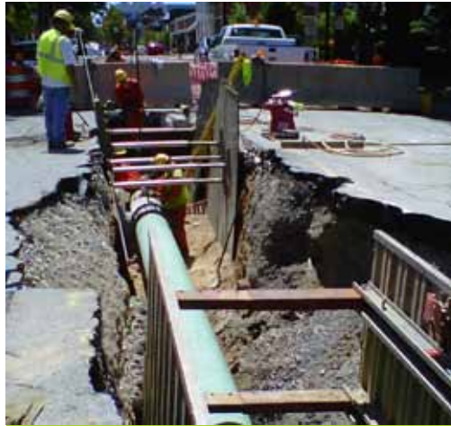
Crews install a 20-inch steel pipeline and a 6-inch plastic pipeline in the same trench along a back alley in downtown York.
