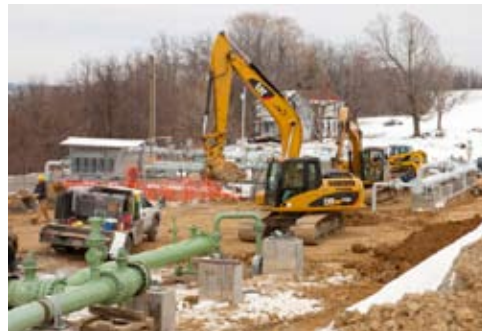
Pictured above is the meter station currently under construction. It is the point where Columbia Transmission (green pipeline) and Spectra (white pipeline) exchange gas ownership
