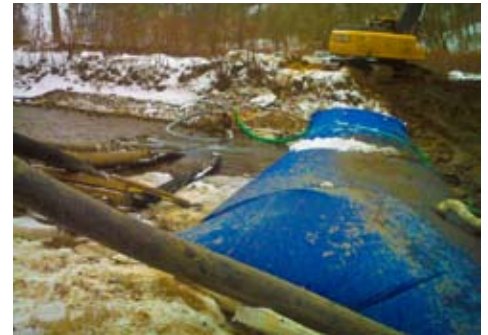
An aqua barrier stops water flow so crews can install the pipeline across the creek.
