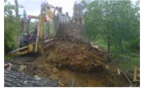
Miller crews assisted Alabama Power with removing uprooted trees from properties where gas service needed to be restored.
