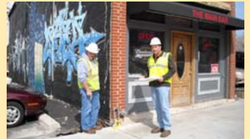
Jim discusses placement of a service on a bar in downtown Columbus, OH with Columbia inspector Bob Cook
