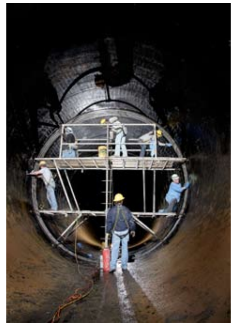
Technicians install a WEKO-SEAL into a 210-inch pipeline. Login to the Miller Hub to see more photos from the project
